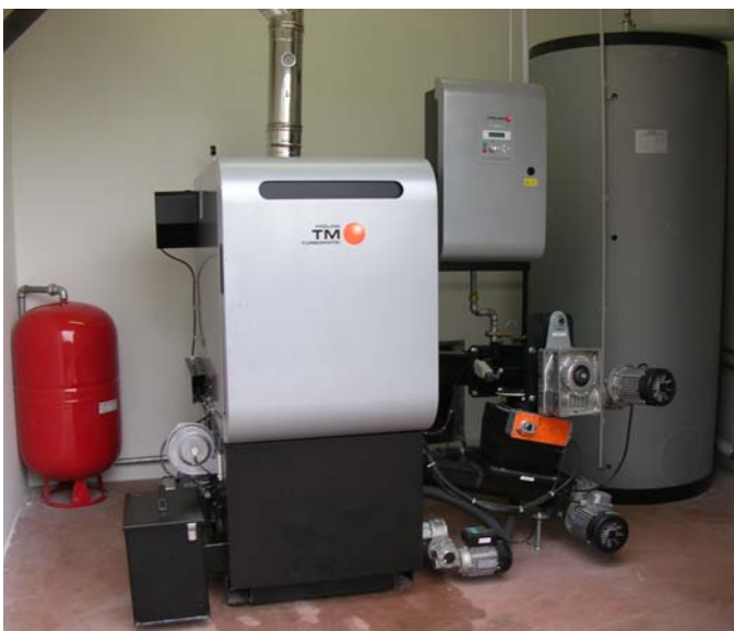
Fig. 3 The biomass boiler
