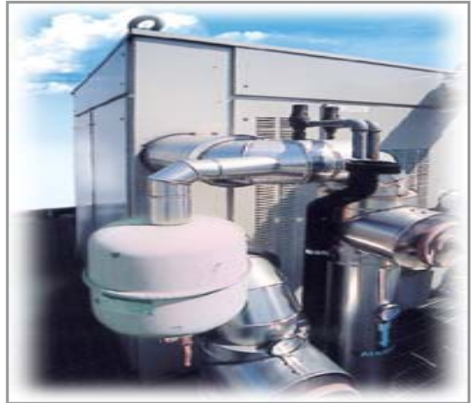
Fig. 4 The absorption chiller
